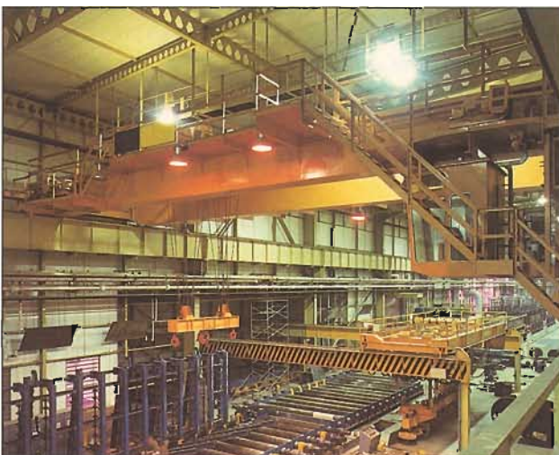
Steel mills. Couplings fitted on 35 tonne overhead crane, and on table roller drives.
